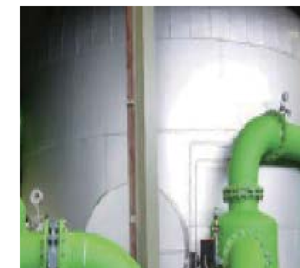
CPP (Condensate Polishing Plant)
