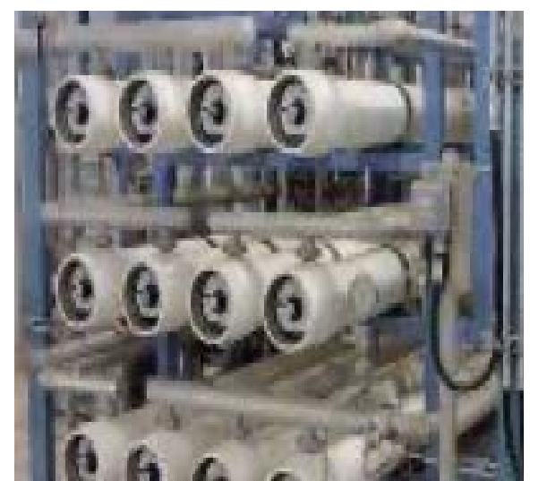
RO (Reverse Osmosis)
